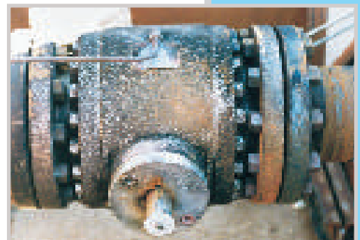
Successfully completed firesafe test.
